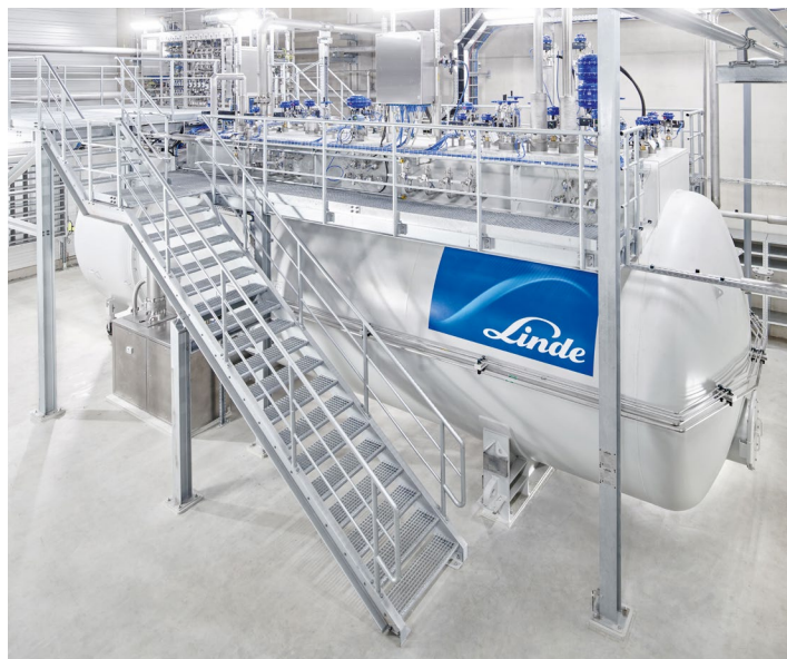
Hydrogen liquefaction plant in Leuna, Germany
