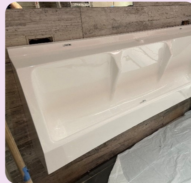
New waterless urinals during the construction/installation of the new toilet block, March 2025.
