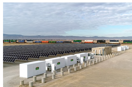
Energy storage facility using EV batteries
