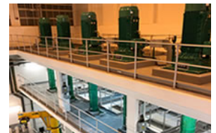
Lusail sewage treatment plant
