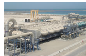
Taweelah B Power & Desalination Complex
