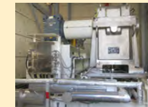
Hydrogen supply facilities at Ariake Bus Depot
