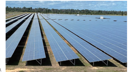
Solar power system installed by SchneiTec Co., Ltd.
