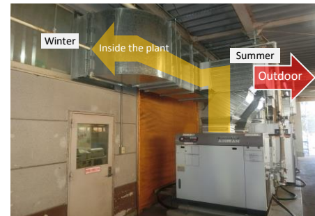
Efficient use of compressor exhaust heat
