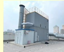
VOC Treatment Equipment
