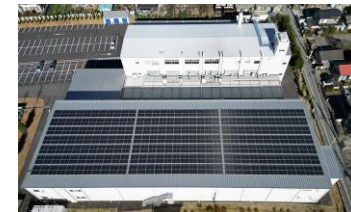
Akagi Plant Solar Power Generation System
