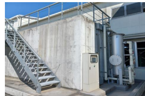
Higashi Nihon Die Casting Industry Co., Ltd. wastewater treatment equipment
