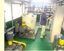
Wastewater Treatment Management Room
