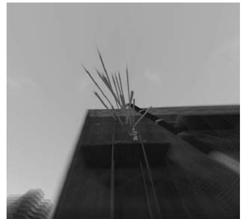
Flying object accident caused by failed crane operation
