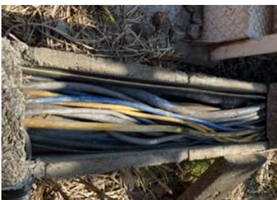
▲Signal cables placed along a track
