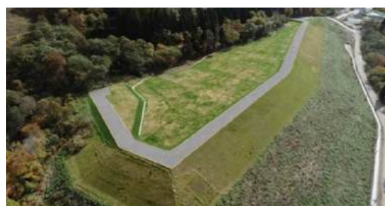
Reinforcement work by soil stabilization at the Yatani Mine Tailings Dam (completion)
