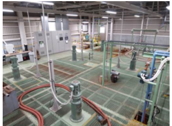
Upgraded pit wastewater treatment facility (Osarizawa Mine)
