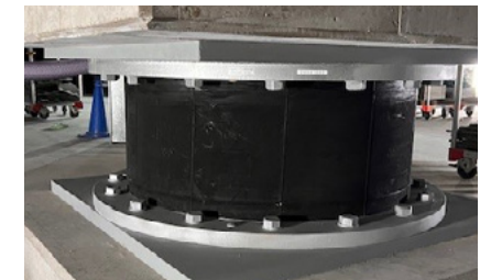
Yaesu Daibiru Building's intermediate seismic isolator
