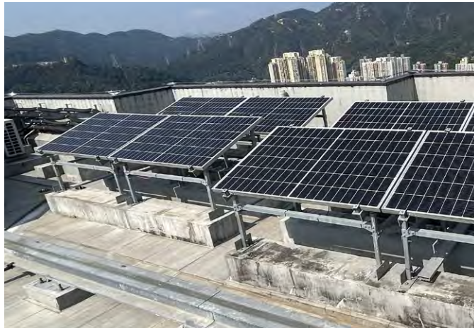
Installation of the solar panels (Left) and wind turbines (Right) at THE PAVILIA FARM
