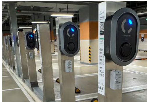
Over 230 parking spaces at THE SOUTHSIDE have been equipped with EV charging facilities, supporting the wider adoption of EVs in Hong Kong
