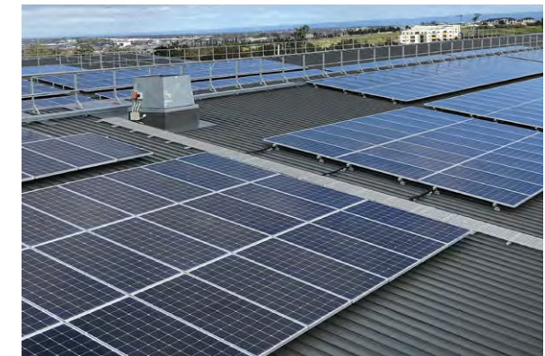
Sydney Metro Trains Facility are equipped with over 3,000 solar panels
