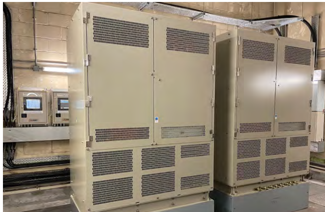
Energy Saving Inverter systems at station
