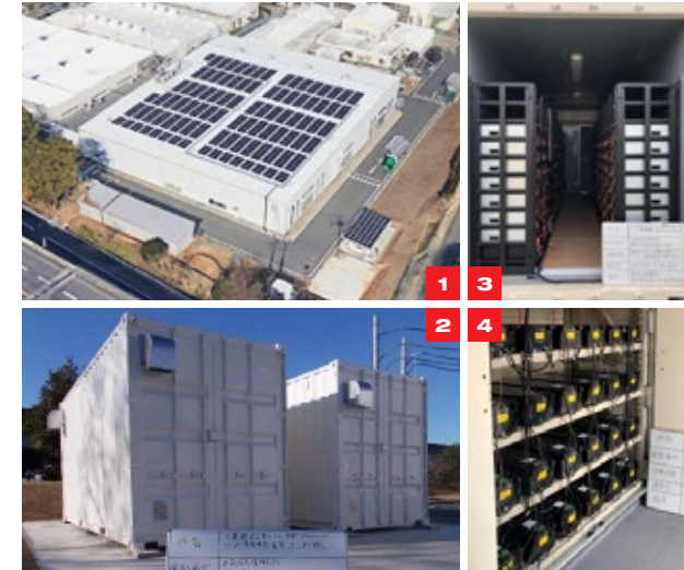
1 Solar panels installed at Head Office and Shin-minami Plant 2 Storage battery container 3 Storage battery 600 kW: Storage battery and HSC are installed inside the storage battery container 4 EMS: HSC24 direct MD / 4x6 standard
