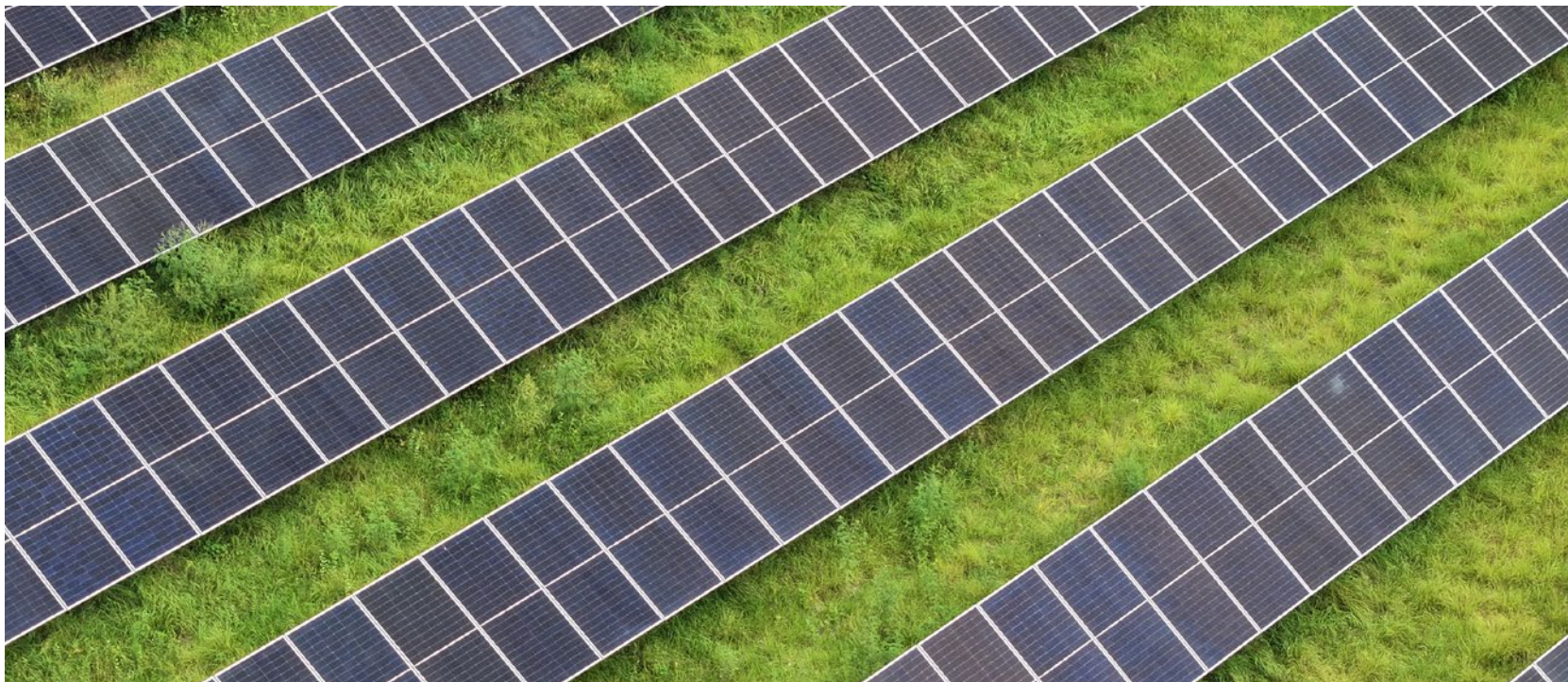
Silver Palm Solar Energy Center in Loxahatchee, Fla.
