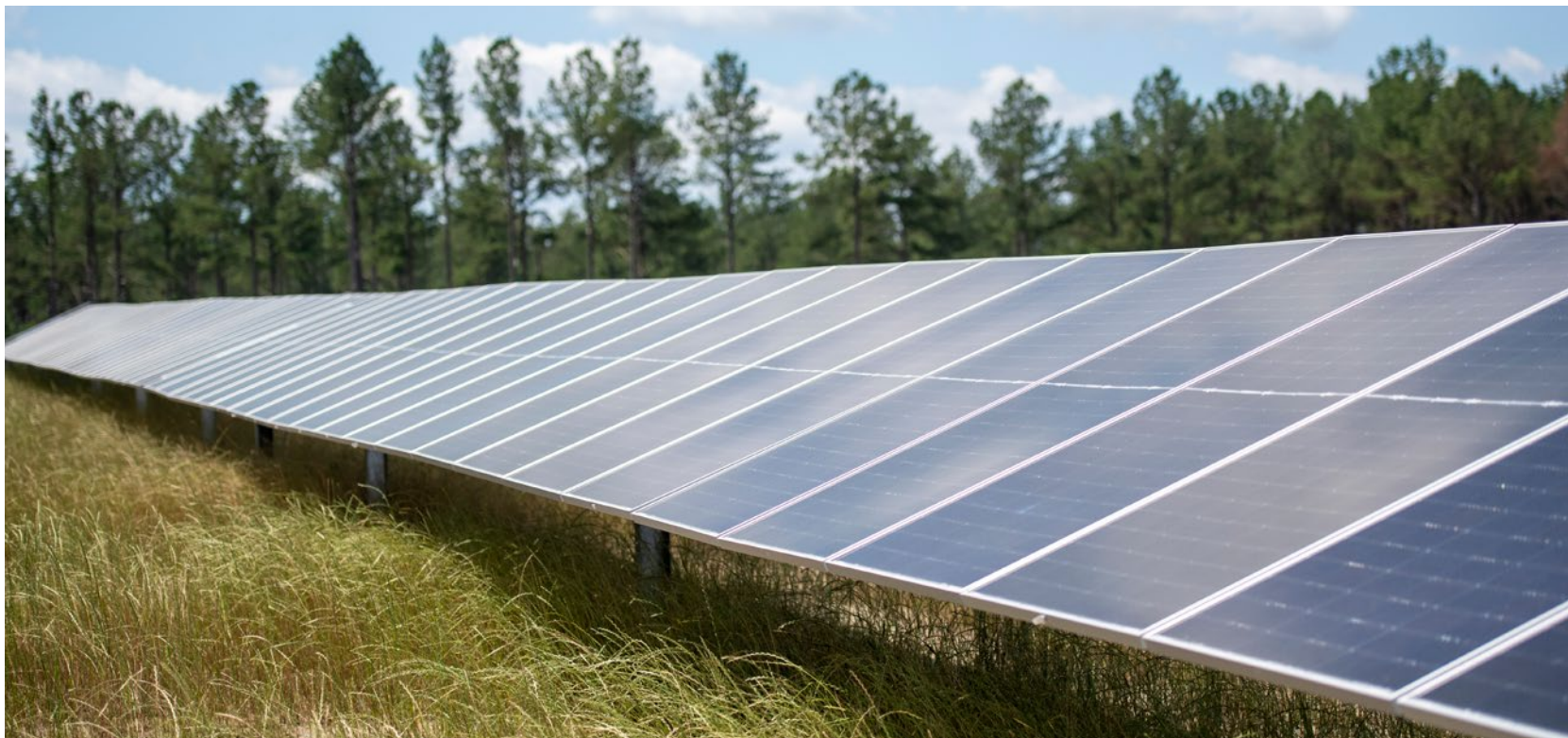
Wild Quail Solar Energy Center in Defuniak Springs, Fla.
