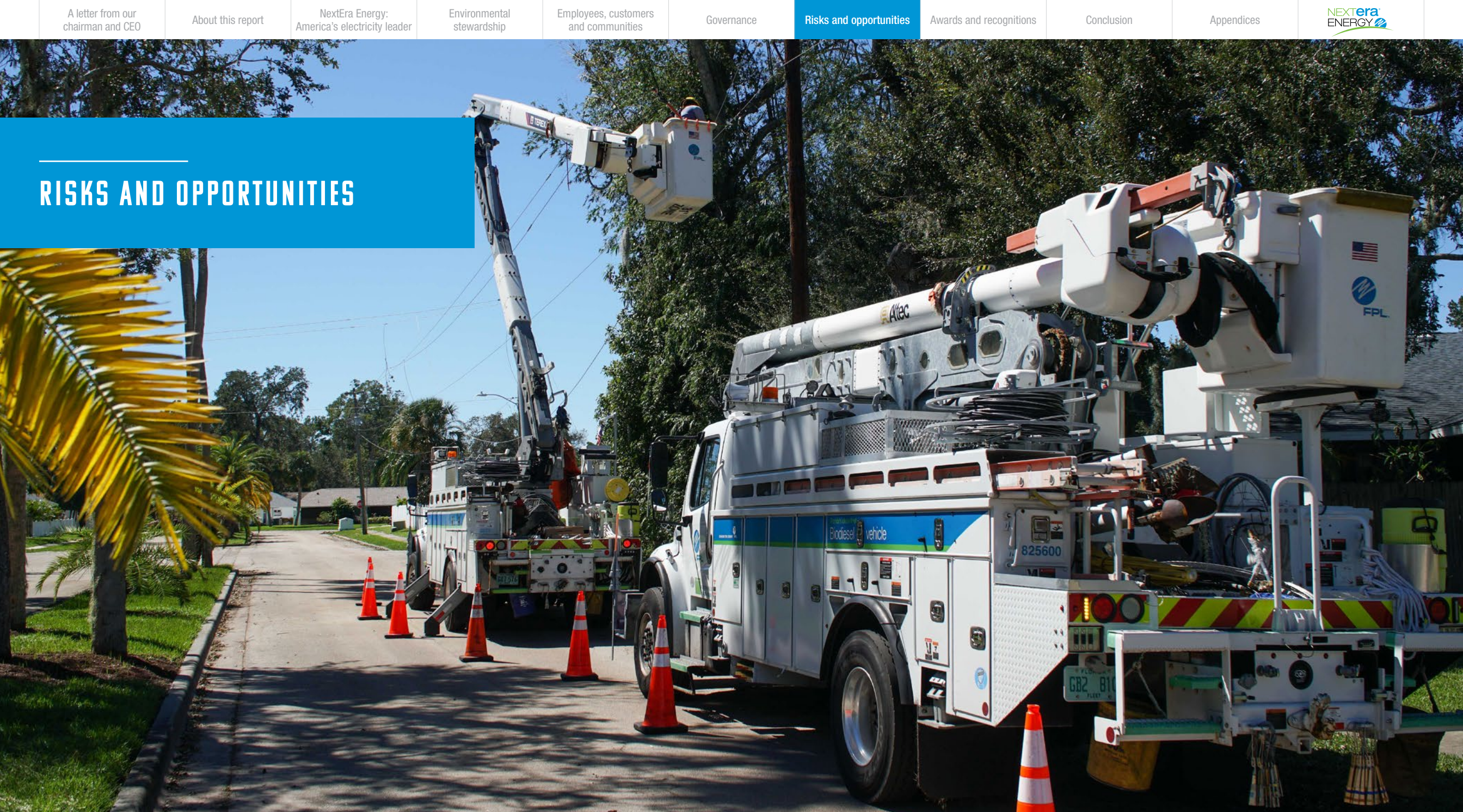
FPL crews work to restore power for customers after a major storm, reinforcing reliability across the grid.
