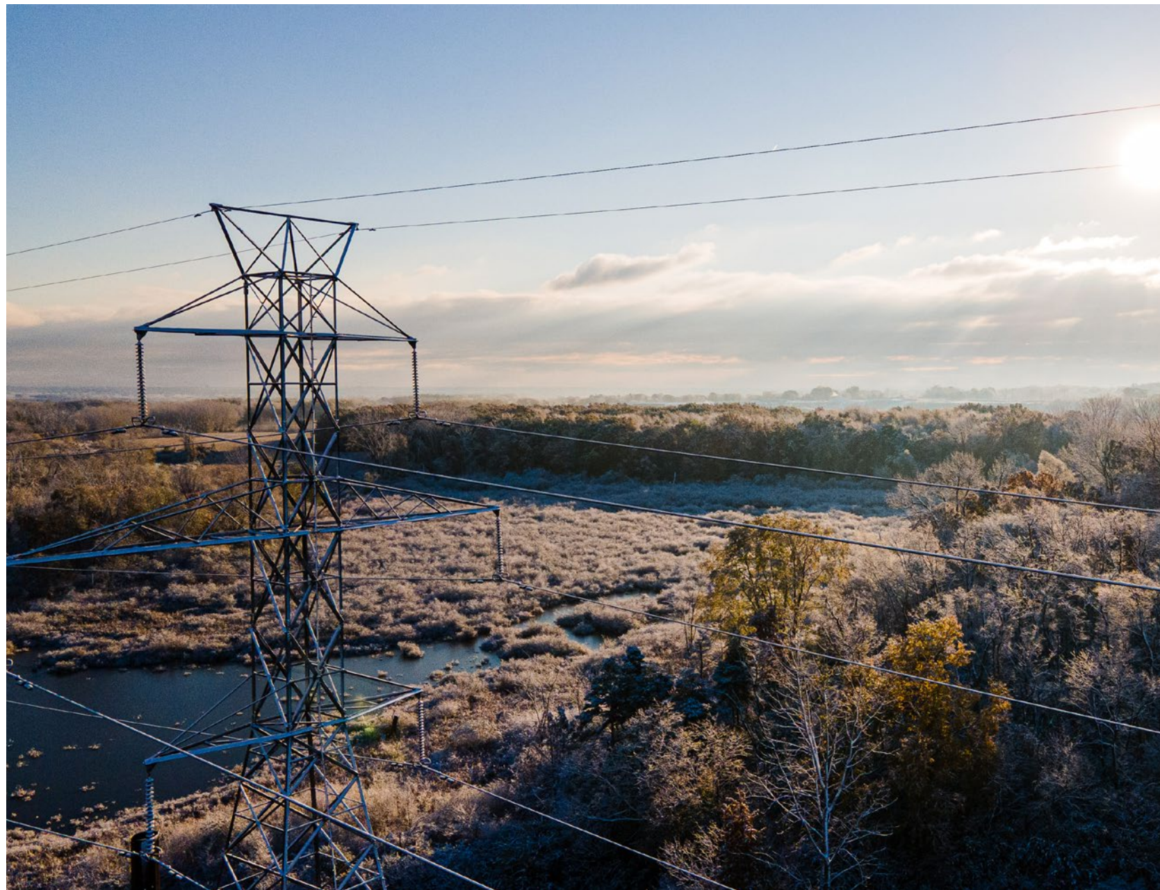
NextEra Energy Transmission MidAtlantic Indiana rebuilt a 20-mile double-circuit overhead 345-kilovolt transmission line.
