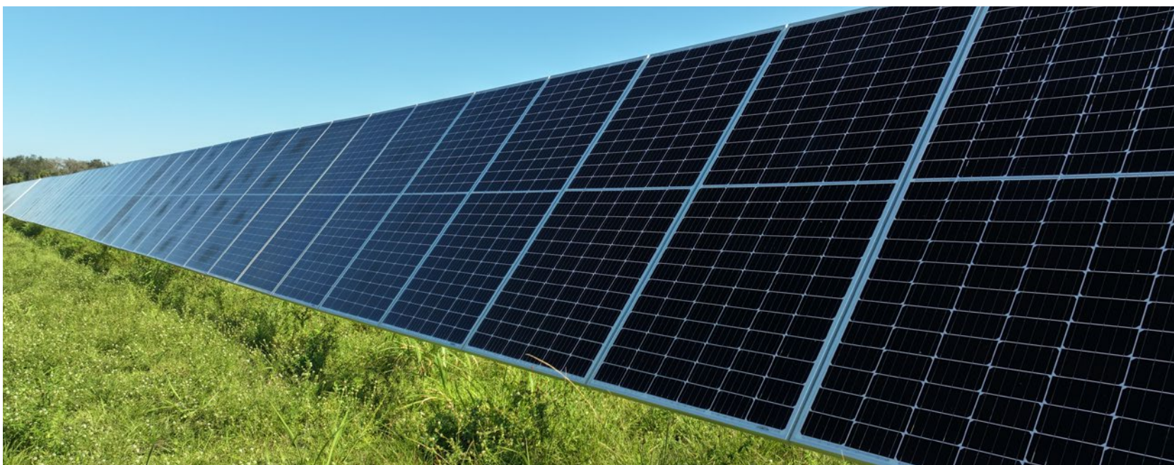
Monarch Solar Energy Center came online in 2023, near the site of a former FPL coal plant in Indiantown, Fla.
