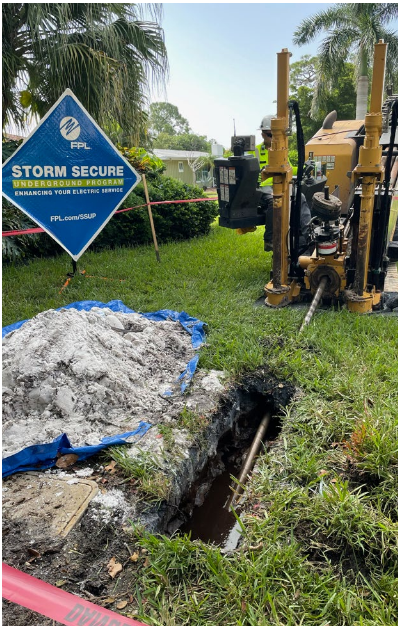
Our storm secure underground program has brought underground power lines to nearly 2,000 neighborhoods throughout Florida.
