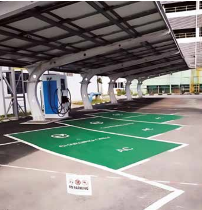
EV charging stations in GTP
