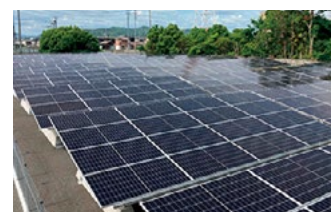
Off-site corporate PPA (Himeji City, Hyogo Prefecture)
