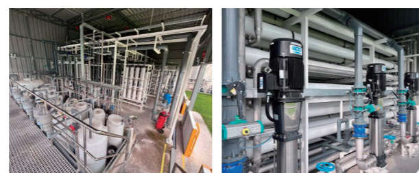
Filtration equipment used in wastewater treatment.
