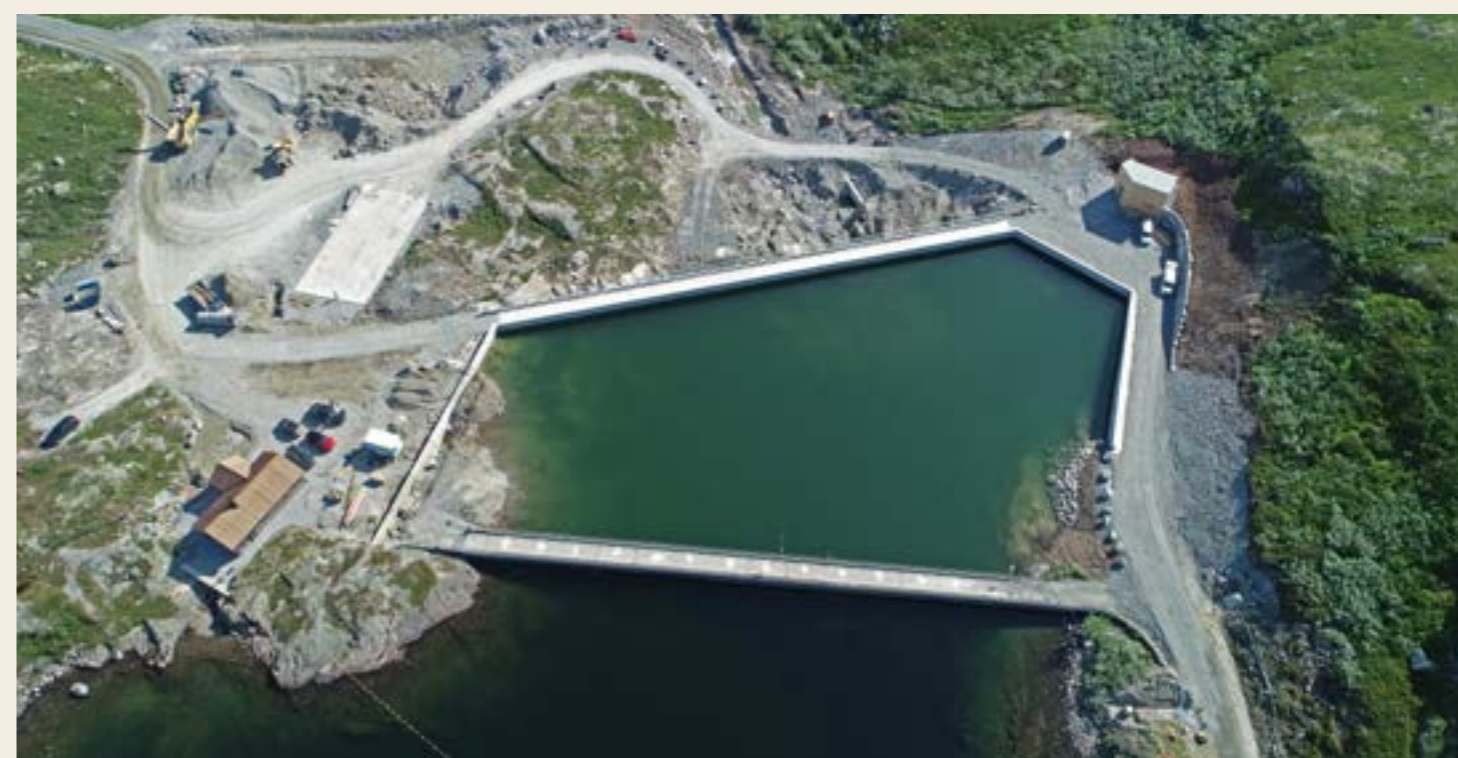
From top left: Holmaneset Green Ammonia | Raskiftet Wind Park | New dam in Mjåvatn, Hallingdal
