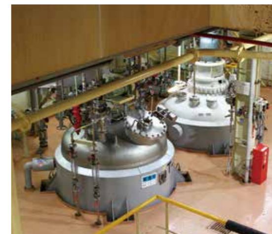
GMP-compliant plant for pharmaceutical manufacturing
