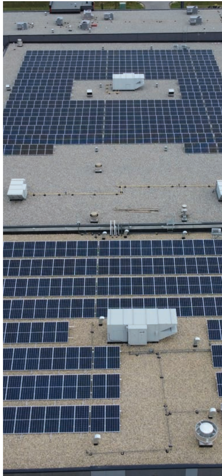
Solar panels at Acheson head office and maintenance facility.
