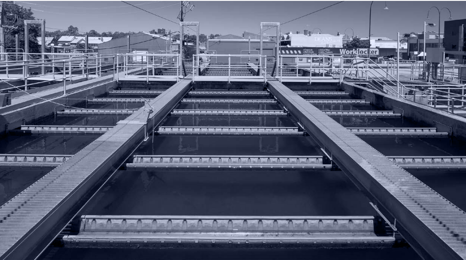
Wangaratta Water Treatment Plant.
