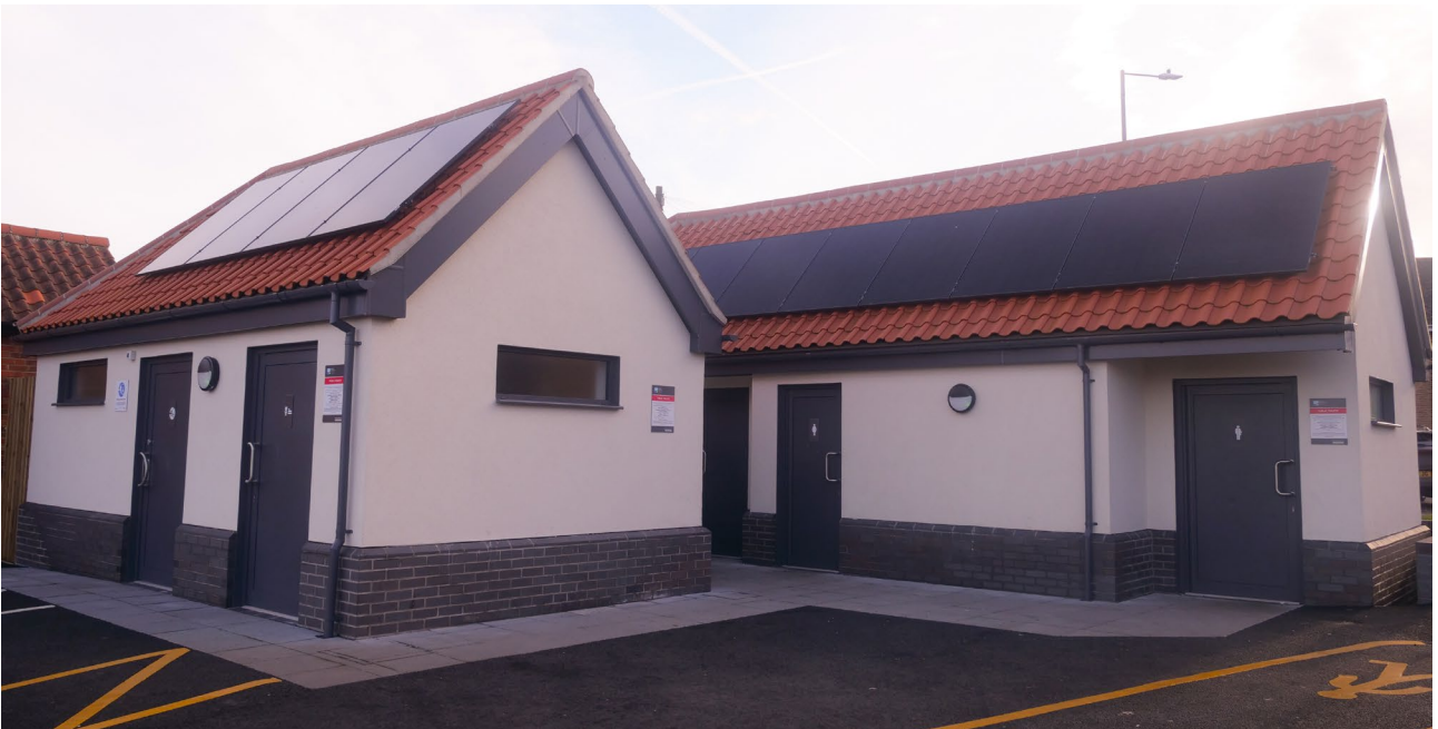
Solar PV on Vicarage Street, North Walsham, toilet block installed in 2023
