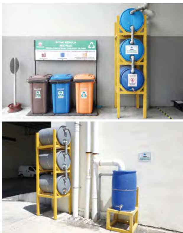
Rainwater harvesting system
