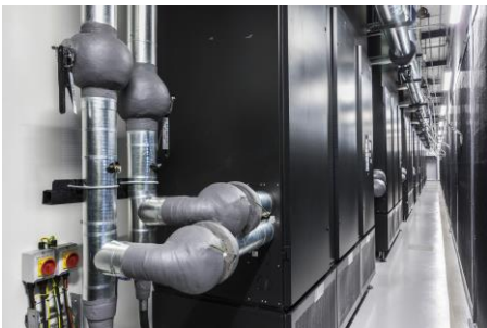
Johannesburg 1 Data Center Johannesburg, South Africa
