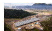
Geothermal power plant under development by Eastland Generation Plant name: TOPP2 Generating capacity: 49MW
