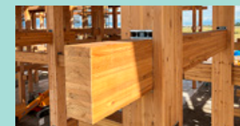
Joints of the Grand Ring. The joints between the pillars and horizontal beams of the structure were reinforced with metal fittings (steel plates and lag screw bolts) for extra rigidity.
