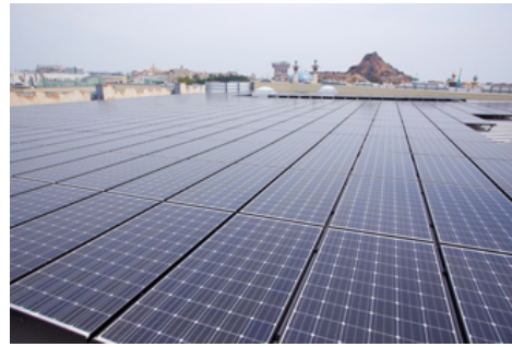
Solar panels installed atop a company building
