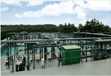
Water treatment facility
