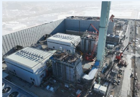
Himeji Natural Gas Power Plant
