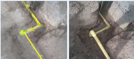
Left: Generated 3D model data (Can be used for construction drawings) Right: Actual installed piping (Recognize required information when taking photographs)
