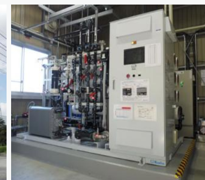
Water purification system with electrical resin regenerator
