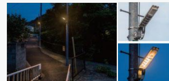
Street lights in Zushi City are replaced with firefly-friendly LED lights
