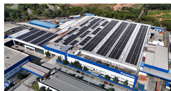
Photovoltaic power generation systems at the Panasonic Appliances Air-Conditioning Malaysia Sdn Bhd.
