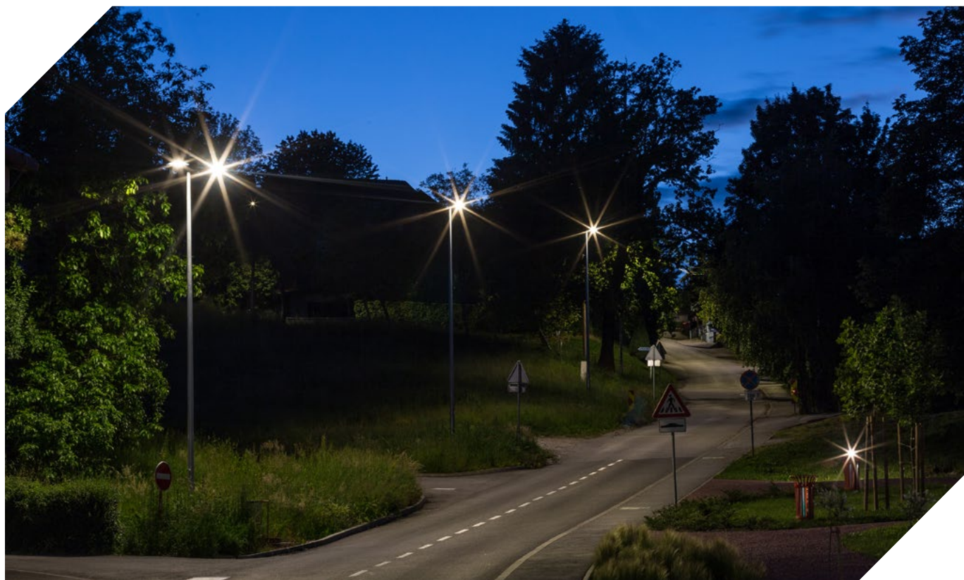
Energy renovation of public lighting by the Petrol Group and savings in 2018-2022 and 2023 plan
