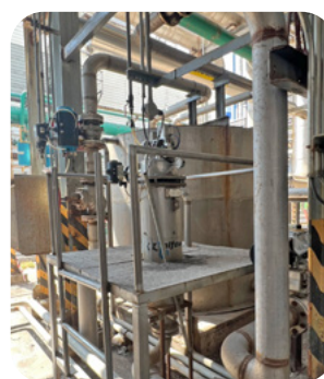
Recycle water - Pump Sealing Siam Kraft Industry Co., Ltd. (Kanchanaburi).
