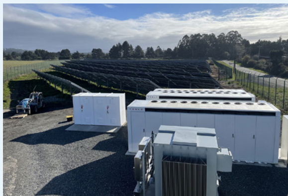
Photo of California's first 100% renewable energy, front-of-the-meter, multi-customer microgrid, which provides enhanced energy resilience for the California Redwood Coast-Humboldt County Airport and U.S. Coast Guard Air Station.
