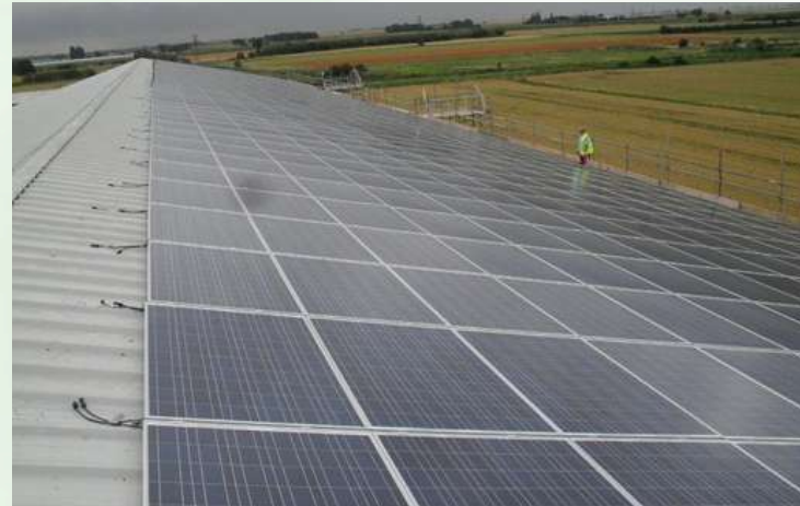
Solar panels installed at our site
