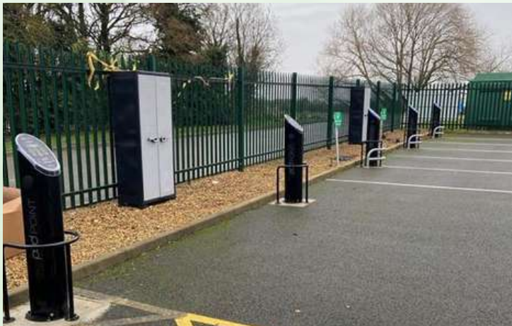
EV charging points at our site
