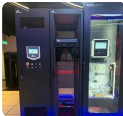
Cutting-edge liquid-cooling technologies
