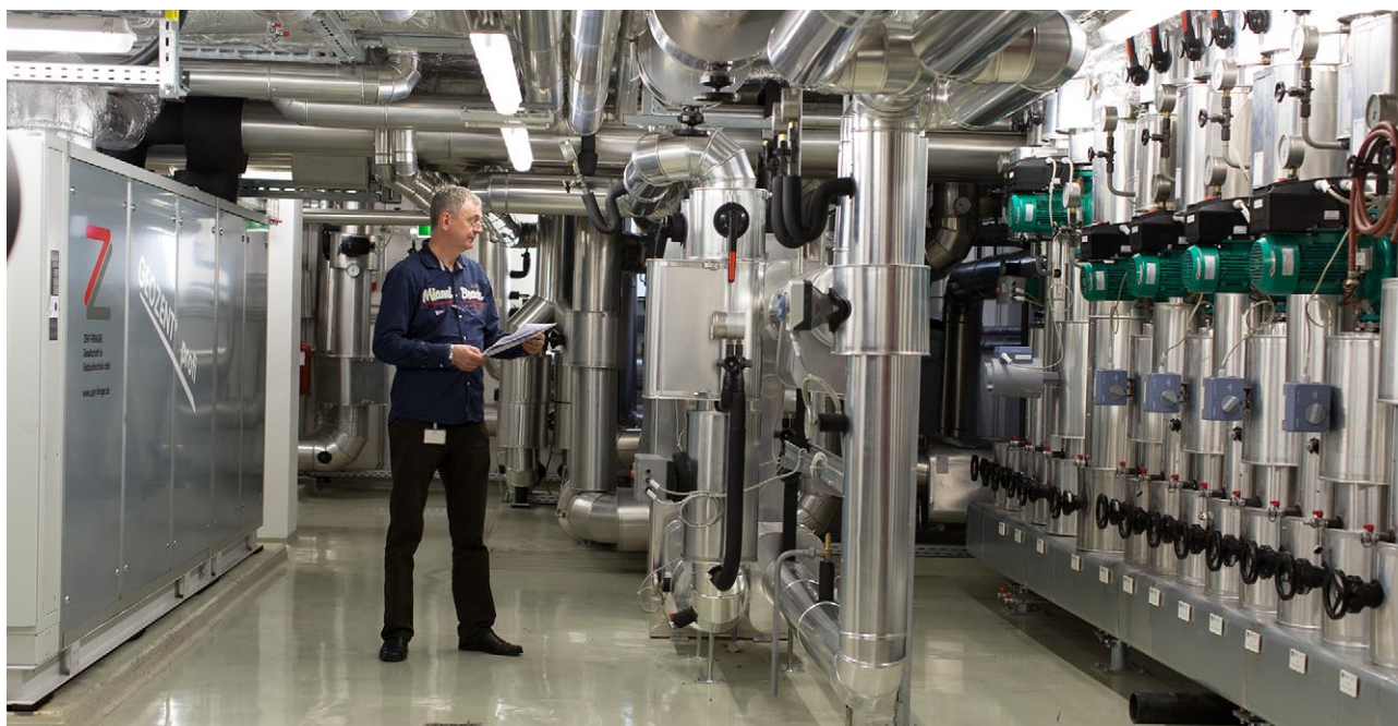
The geothermal system heats and cools the R+V office building in Wiesbaden.
