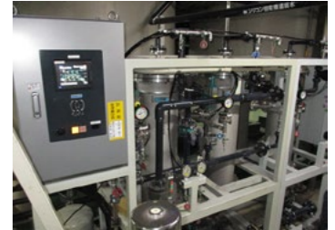
Membrane Filtration Facilities
