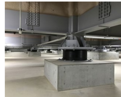
Adoption of Seismic Isolation Structure Including Ancillary Areas (ROHM Apollo Chikugo Plant)
