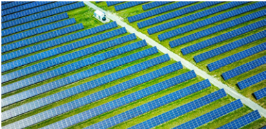
Solar Power Projects in the T&I Group
