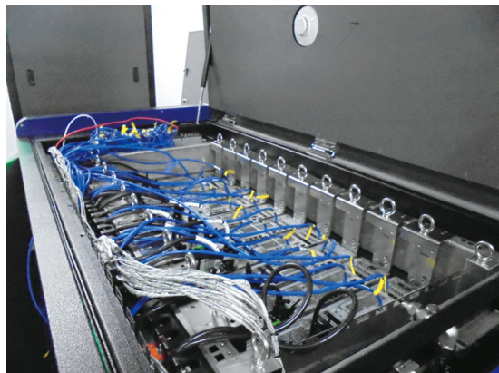
Server with Immersion Cooling Technology
