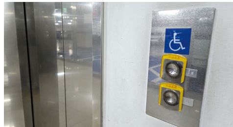
Elevators for Persons with Disabilities
