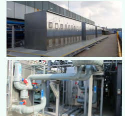
Nitrogen oxide treatment facility
