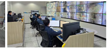
Security Control Room
