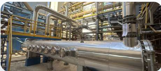
Technology to reduce water consumption and enhance efficiency based on the 3R principles.
