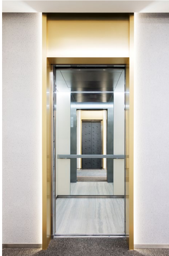
A modernized elevator, upgraded and ready for use at the V Tower
