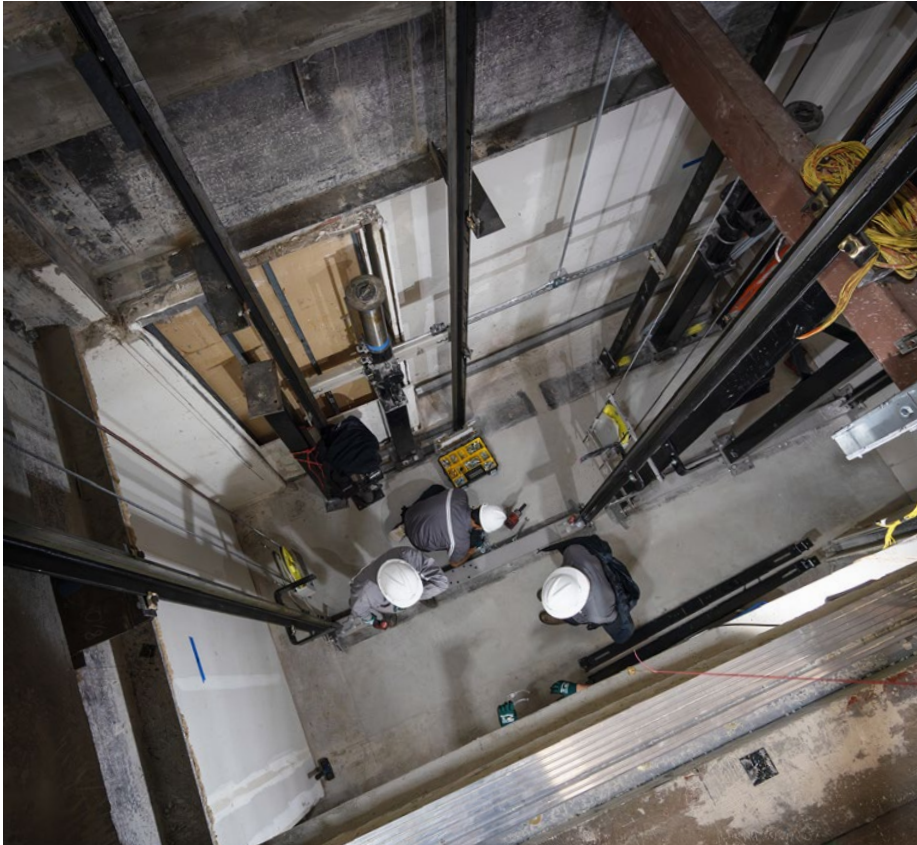
The elevator now extends one floor below where it used to stop.
