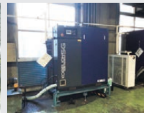
Ironworks compressor (replacing equipment with high-efficiency models)
