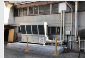
The new chiller
