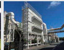
Woodworking dust collector (replacing equipment with high-efficiency models)
