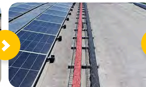
DC string cabling
