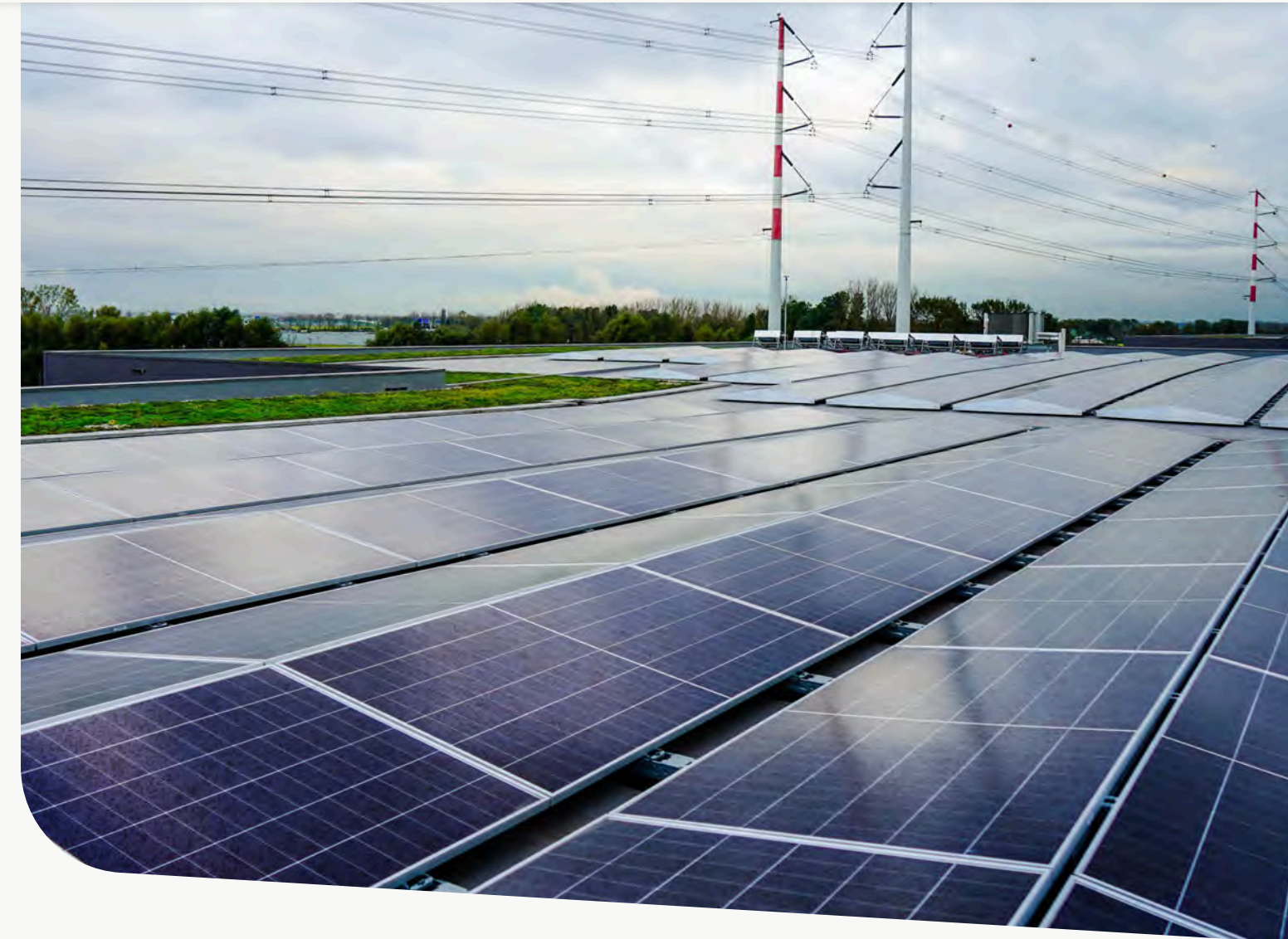
Sunrock Halfweg rooftop solar system (capacity of nearly 2 MWp)
