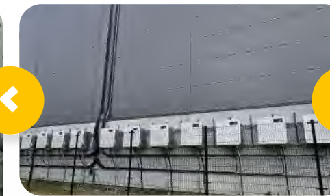
Inverters (installed on a facade)
