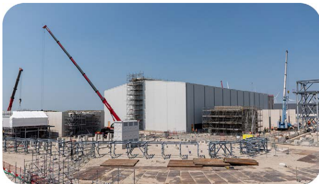
Photo: Holland Hydrogen I, one of Europe's largest renewable hydrogen plants, under construction in the Netherlands.
