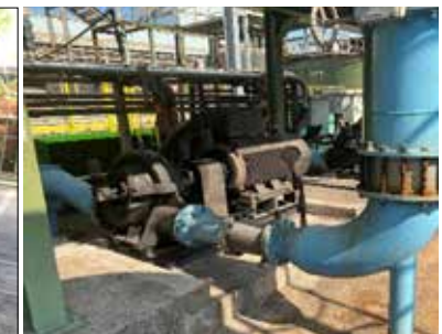
UTL CT-901 cooling water tower coolingfan drive motor energy saving
