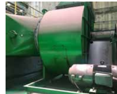
CR2 exhaust fan improvement
