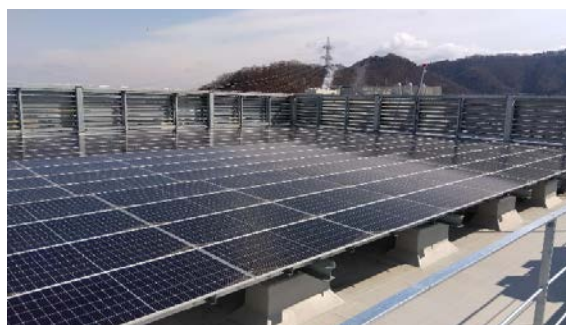
(Chikuma Plant (Chikuma City, Nagano Prefecture))
