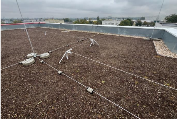
Brown roof on our new store in Germany: Charlottenburg. The vegetation absorbs rainwater to lower quantities reaching the sewer.
