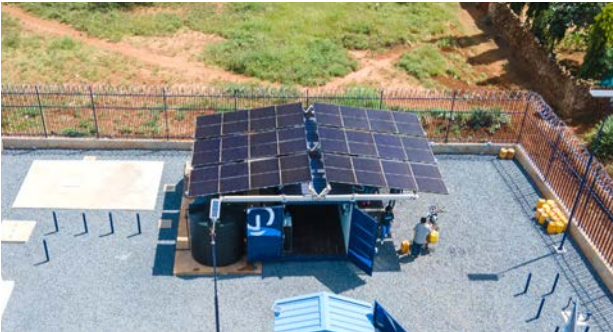
GivePower - Makindu Solar Water Farm Mobi+, Kenya
