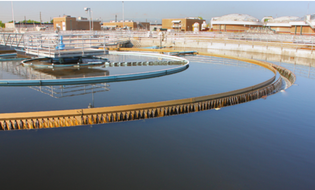
Littleton/Englewood Wastewater Treatment Plant
