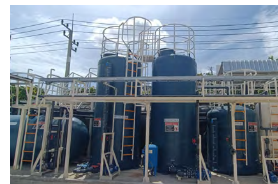
Wastewater treatment recycle plant installed at STT
