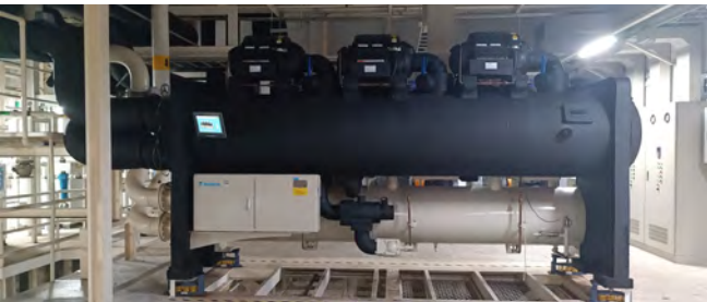
Chiller system installed at STT
