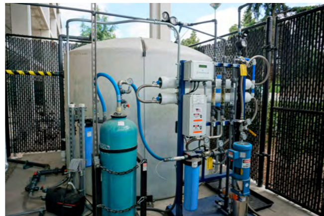
Groundwater treatment system installed at Sony Electronics San Diego
