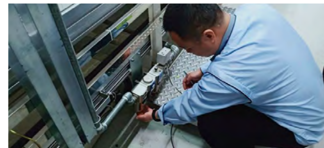
Preventing leakage of high-pressure air to reduce energy consumption at Shanghai Suoguang Visual Products Co., Ltd. (SSVE)
