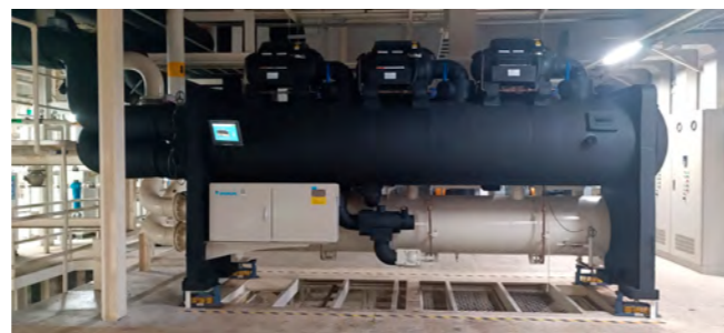
Chiller system installed at STT
