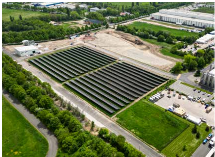
On the factory premises in Ohrdruf , Storck has installed a photovoltaic system with an area of more than 16,000 square metres.
