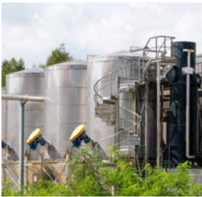
At the Halle location, we purify the process waste water in our own plant.
