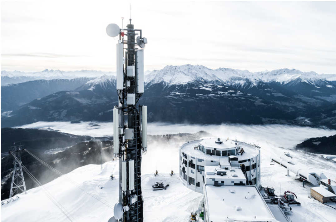
Sunrise antenna site in Laax
